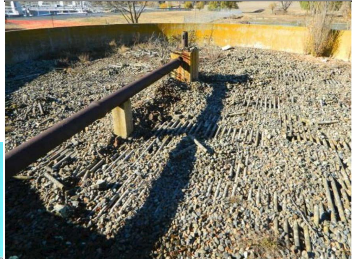
Sewage Treatment Plant, Confidential Site
